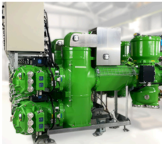
Schakelstation, bron: GE Vernova
