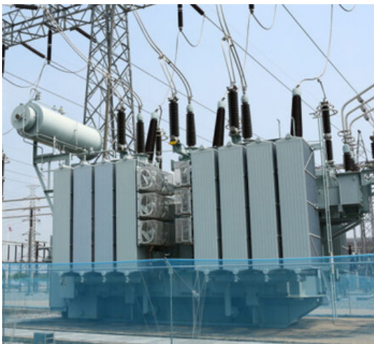
Transformator, bron: Transformers Magazine
